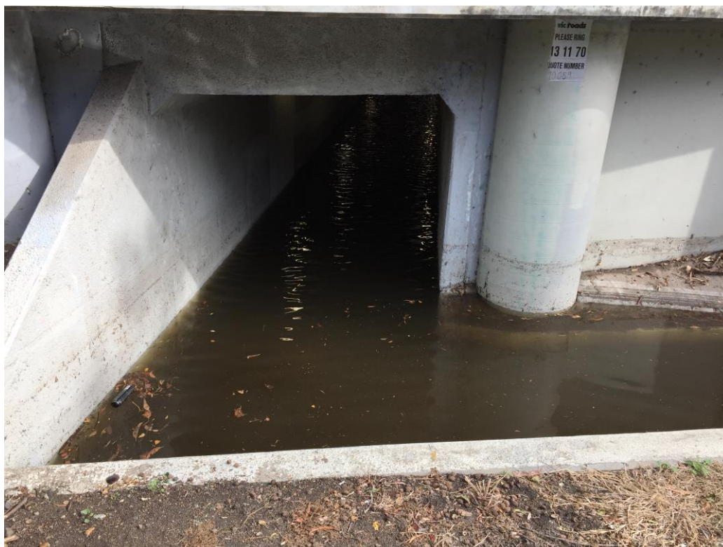
Figure 7. Deeply flooded pedestrian underpass beneath CityLink to access Wheeler St
